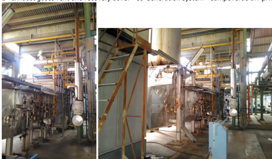
Figure 1 - Exhaust gases vent and recovery boiler - Co-Generation System - Campoverde di Aprilia Plant
