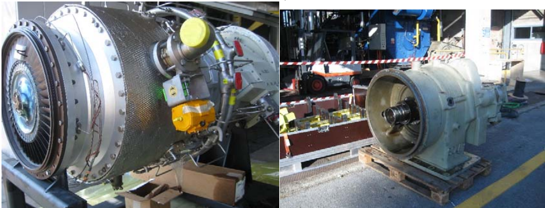
Figure 2 - The gas turbine during its replacement (left); the dismantled reduction gearbox during installation (right) (August 2016)
